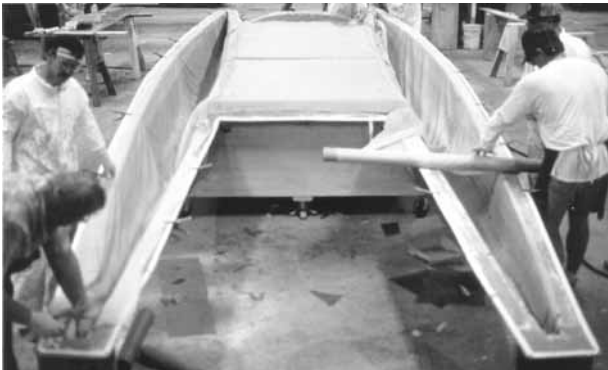
Figure 4-4 After applying an inner layer of fiberglass cloth, release fabric is placed over the laminates.
